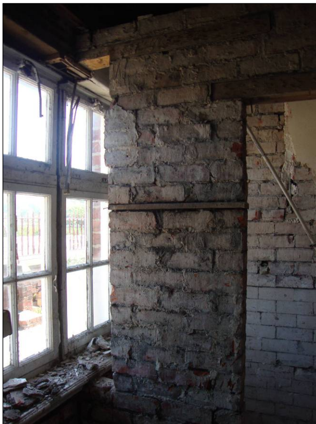
Figure 35: North elevation of Room 2, looking east and showing the detail of the later inserted partition wall.
