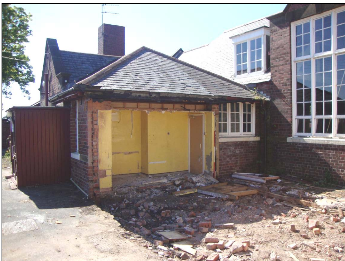
Figure 25: External west facing elevation of Room 11, looking south east and showing where the toilet block has been demolished. Scale = 2m
